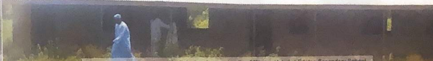
Constituency Project of Hon. Y.M. Esheti under construction 90% completed at Edetso Secondary School.
